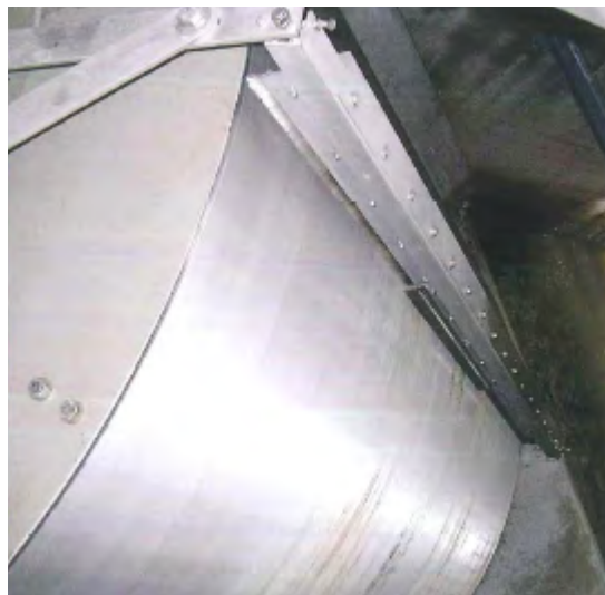
Figure 8.3 Rotary screen of the fine screen installation
